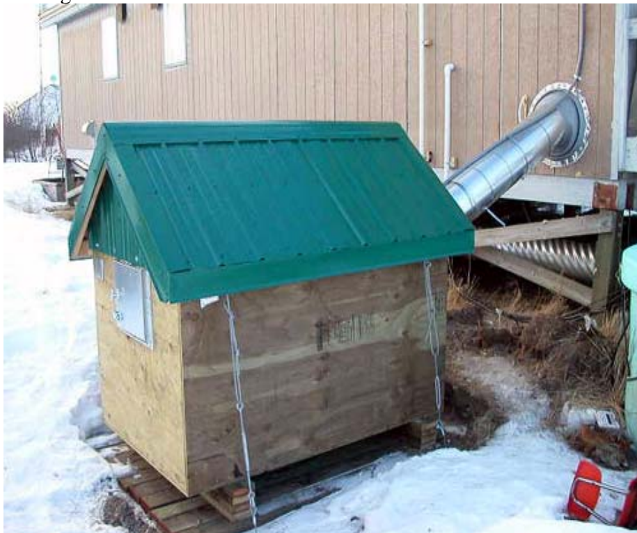
Photo 1: Sewage Holding Tank with metal roof. Note also the metal clad sewage discharge pipe and electrical conduit coming from the building. The hold down cables are used in flood risk locations
